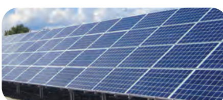
The PVREA Solar Farm (Courtesy of fortcollinscommunitysolar.com )
