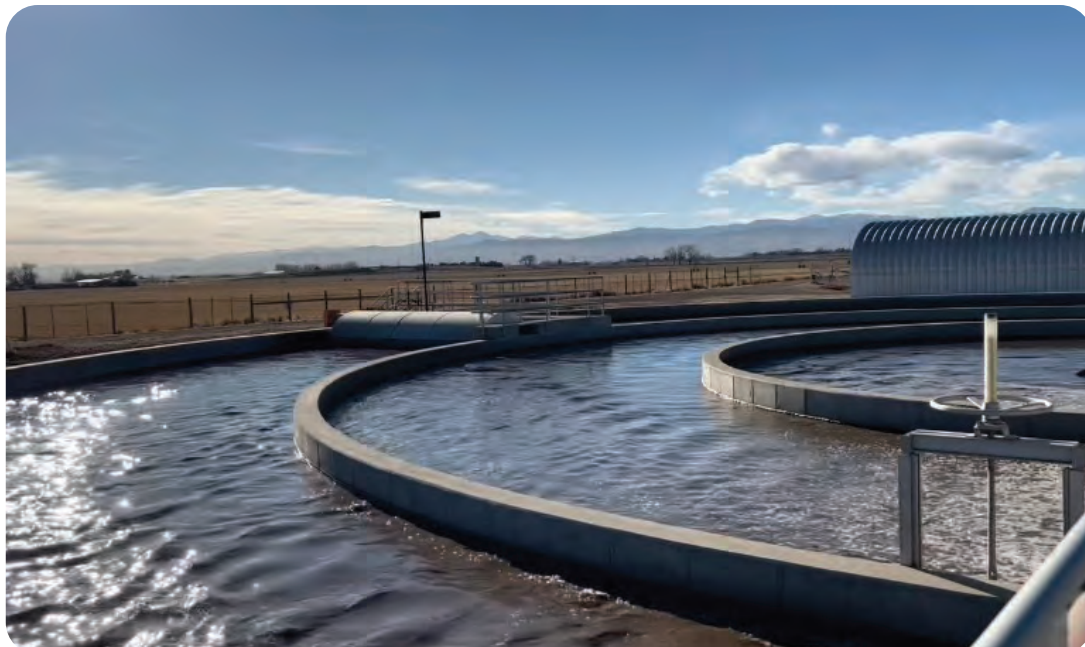
Wellington's wastewater plant (Photo courtesy of Town of Wellington)
