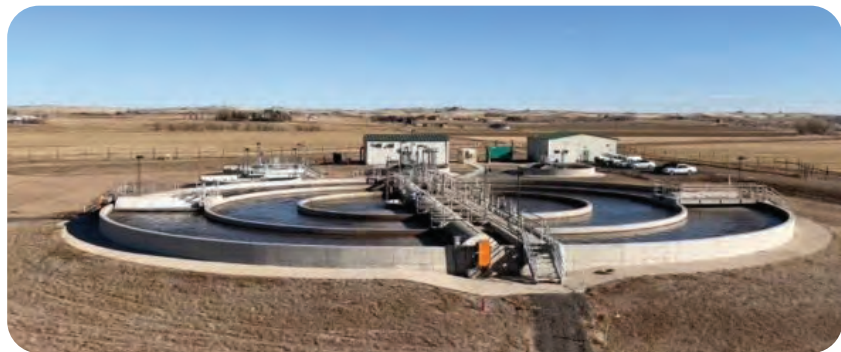
Wellington's wastewater plant (Photo provided by Town of Wellington)
